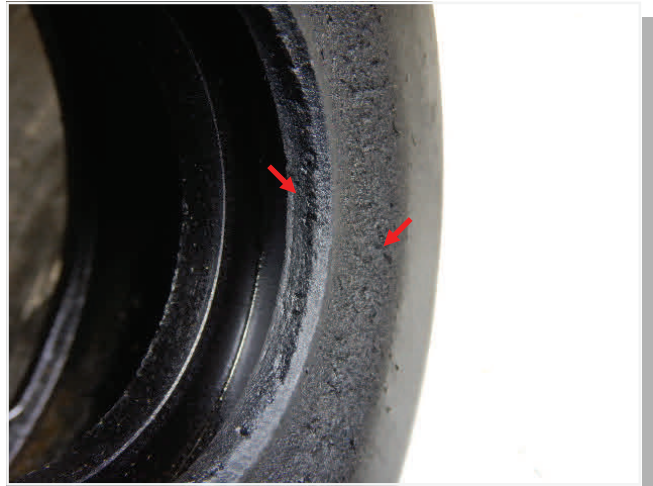
Ph (2) - MUX-FH-Seal Retainer - Replaced - Front face worn close to seal groove.
