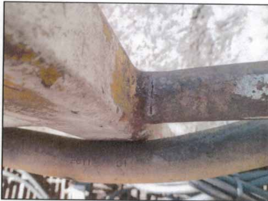
Crack detected on basket, frame shall be repaired.
