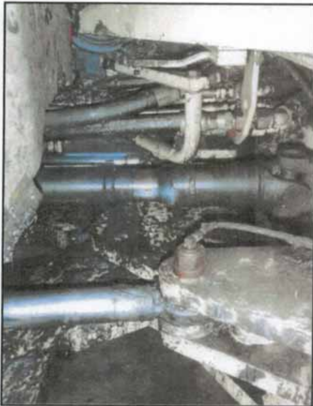
Repair minor hydraulic oil leaks.
